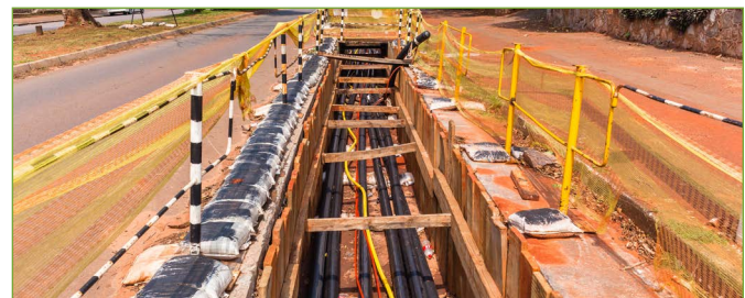
Strategic undergrounding of powerlines can greatly reduce the risk of wildfires in impacted areas.
