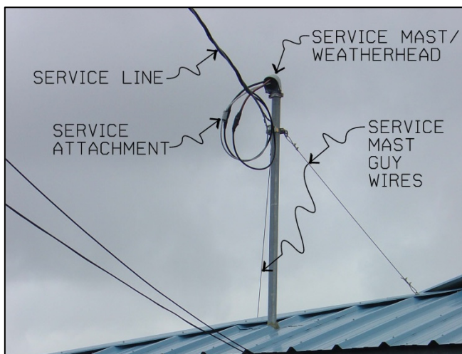
Service attachment at mast/weatherhead
