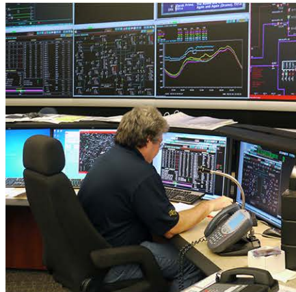
Hawaiian Electric recently upgraded its Energy Management System, the “brain” that controls the electric system.
